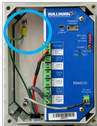
Ground Connection on Remote Monitoring Unit
