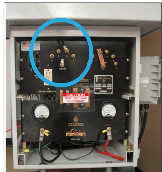
AC Normally Closed Solid State Relay Connected to Rectifier Taps
